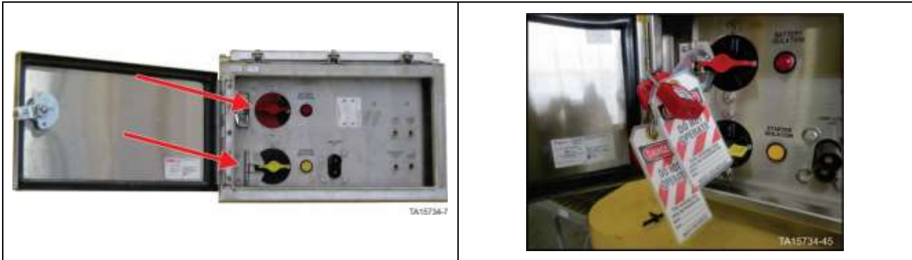
Battery Isolation Box – Battery isolation switch in OFF position with locks in place
