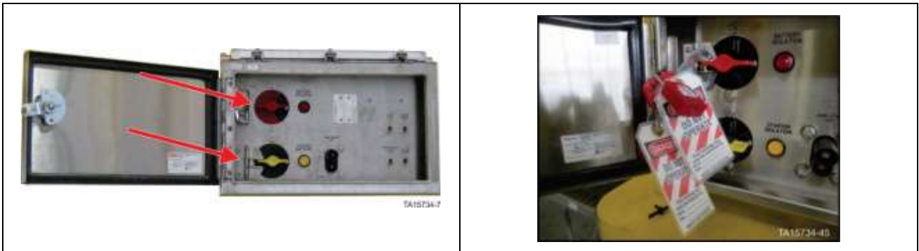
Figure 7. Battery Isolation Box – Battery isolation switch in OFF position with locks in place
