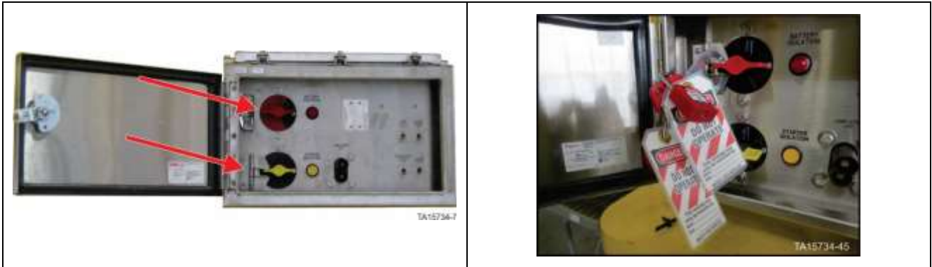
Battery Isolation Box – Battery isolation switch in OFF position with locks in place
