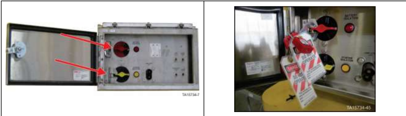
Battery Isolation Box – Battery isolation switch in OFF position with locks in place
